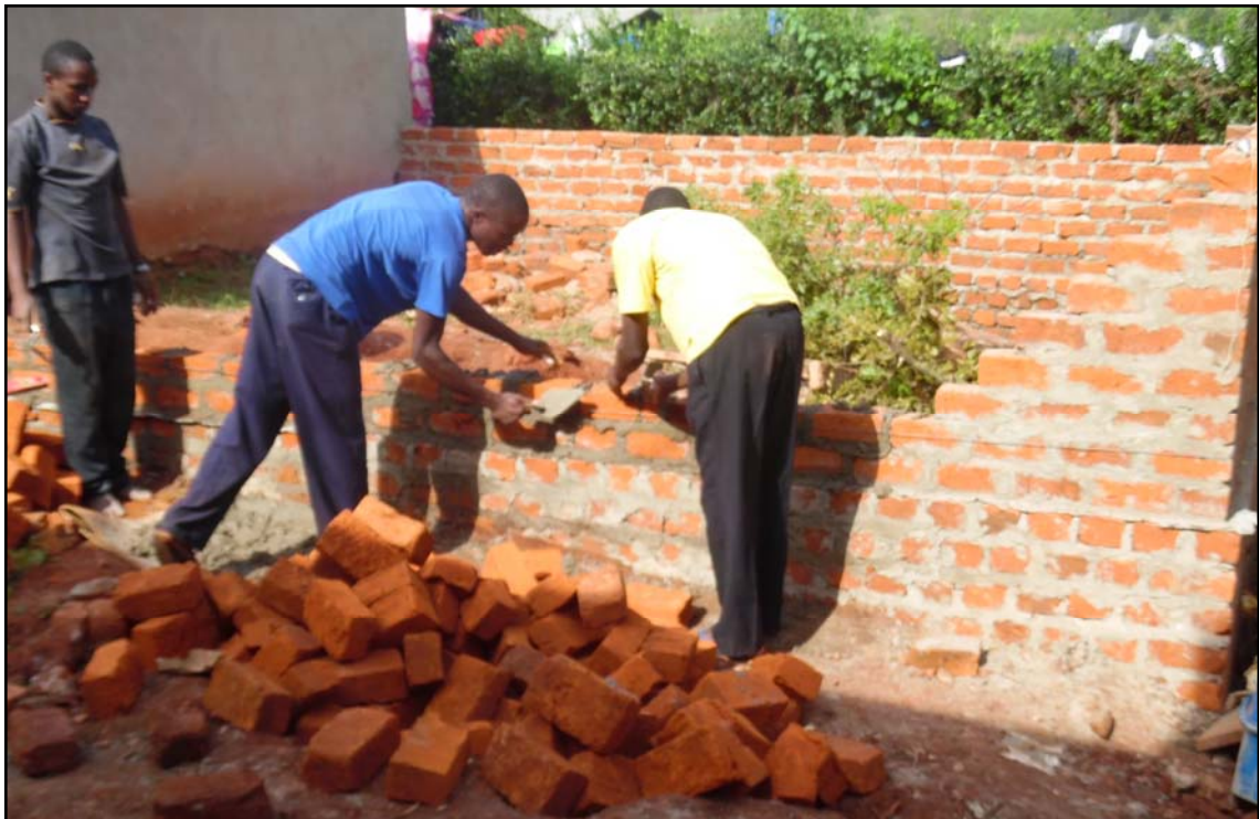
Building and concrete practice students of S.3 constructing a poultry house at the school
